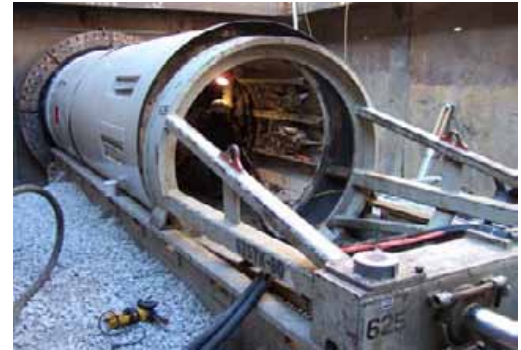
Tunnel Boring Machine - 72-inch diameter pipe crossing under BNSF Railroad & Hwy No. 6
