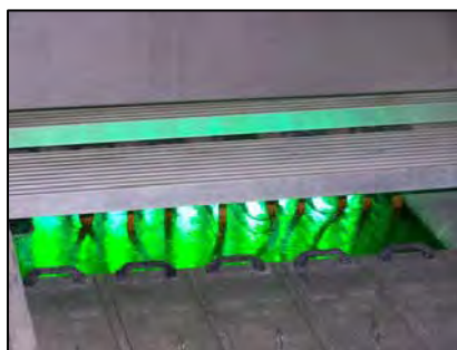
Ultraviolet Disinfection Channel
