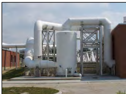
Odor Control Facilities
