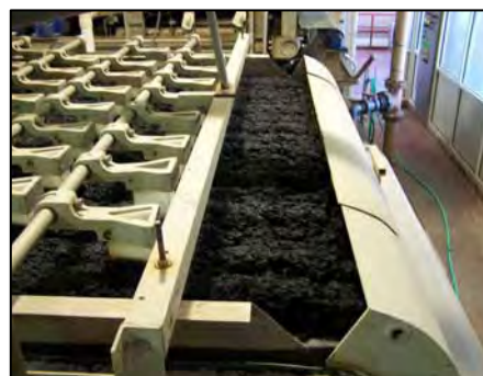
Belt Filter Press Dewatering
