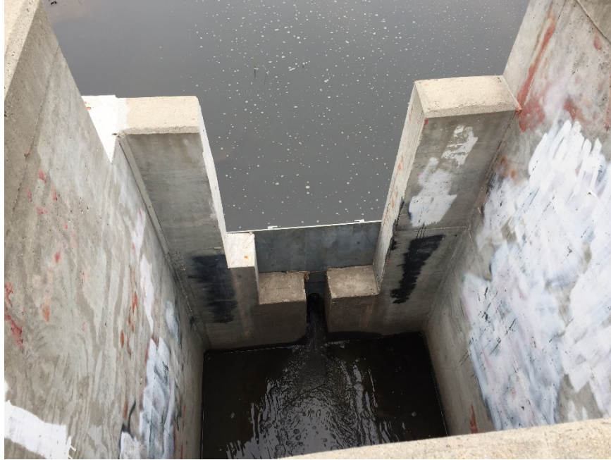
Detention Basin utilizing orifice plate to control discharge
