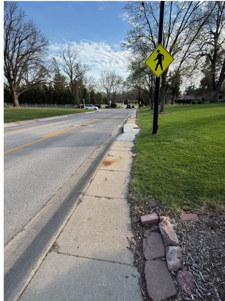
North to south view of S Cotner Blvd – access to Valley Rd. The sidewalk sits directly next to the roadway and is uneven, narrow, and misaligned, creating potential safety hazards for pedestrians.
