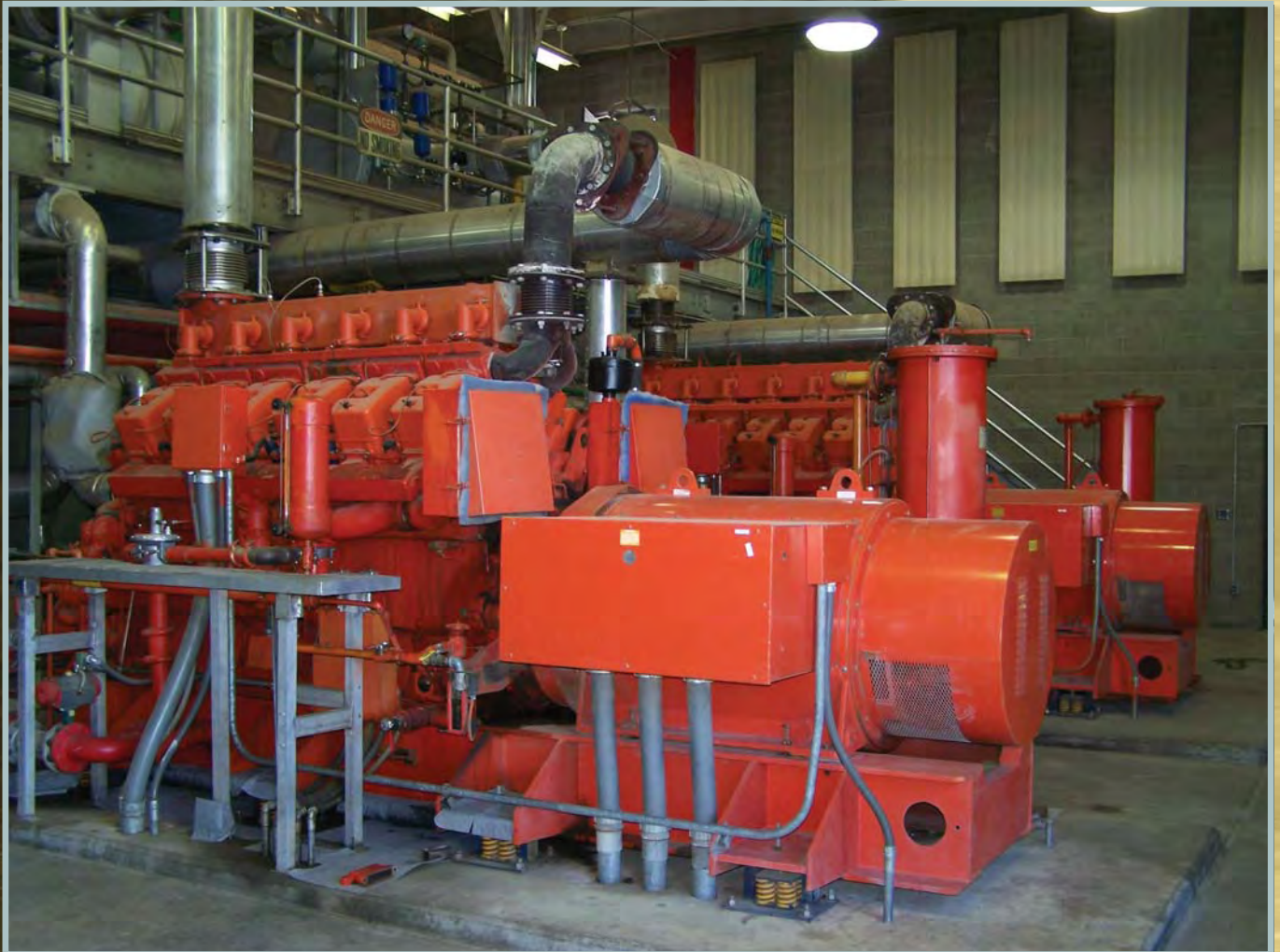
Theresa Street Methane Fired Generator
