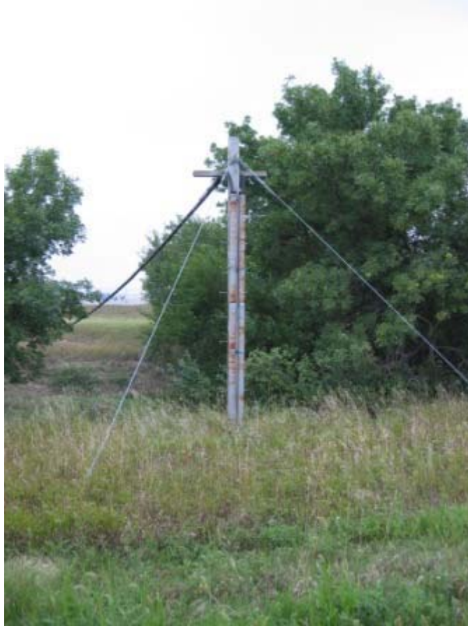
Photo 20. Oak - Communication line from abandoned radar tower viewed from levee road
