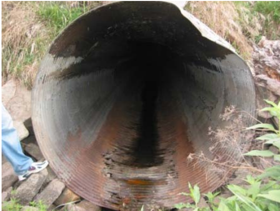
Photo 15. Oak - Air Force Base local drainage culverts US face at levee road - one barrel
