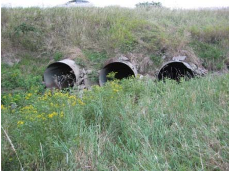
Photo 16. Oak - Air Force Base local drainage culverts US face at levee road
