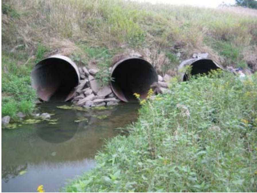
Photo 14. Oak Site - Air Force Base local drainage culverts US face at levee road
