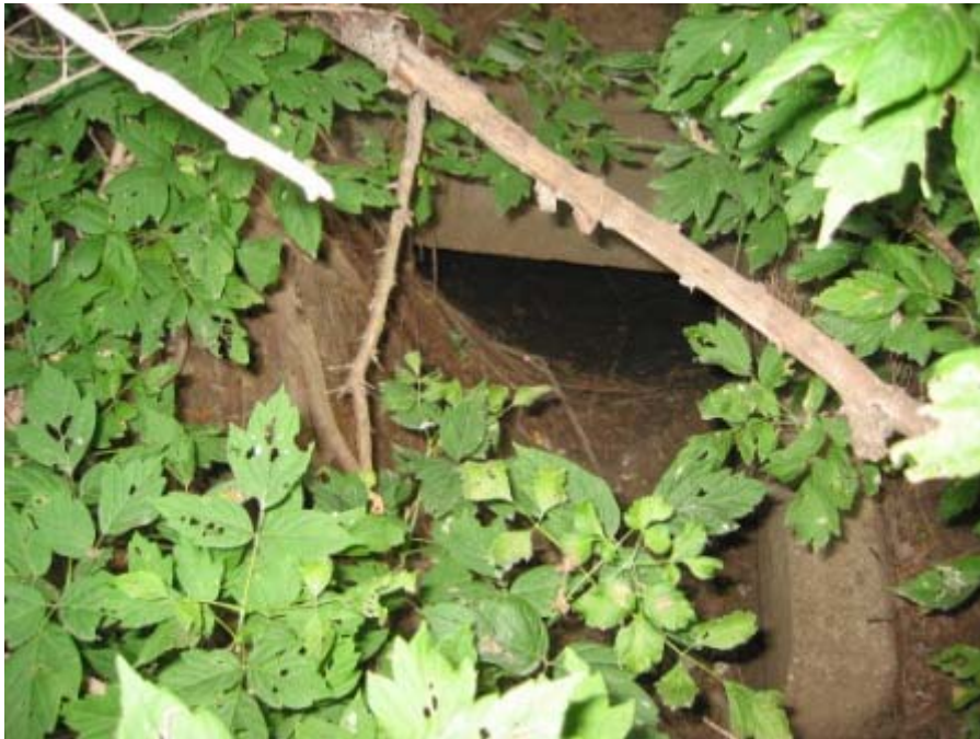
Photo 2. Middle Site - Box culvert, silted in
