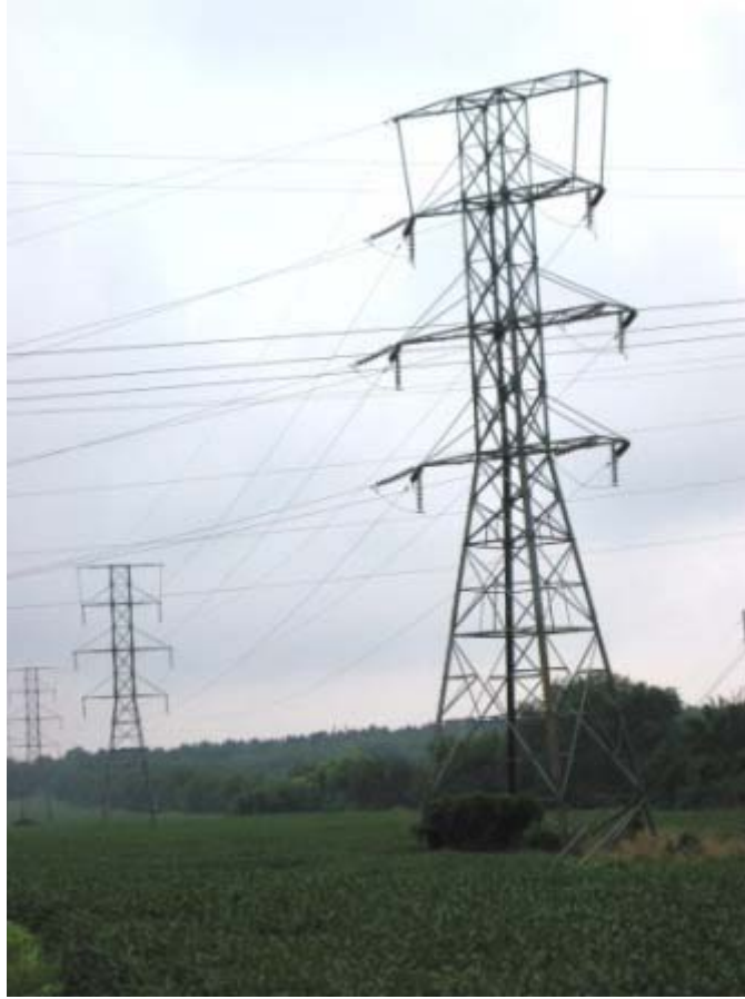
Photo 32. Oak - Start of power line stations on RB from the north
