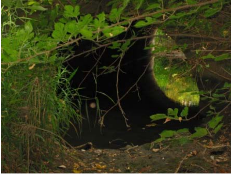
Photo 1. Middle Site – 5-foot Culvert just past VFW on A Street, silted in
