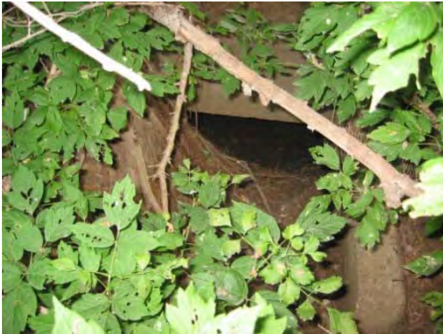
Photo 2. Middle Site - Box culvert, silted in
