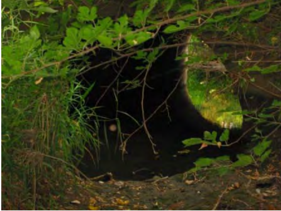
Photo 1. Middle Site – 5-foot Culvert just past VFW on A Street, silted in
