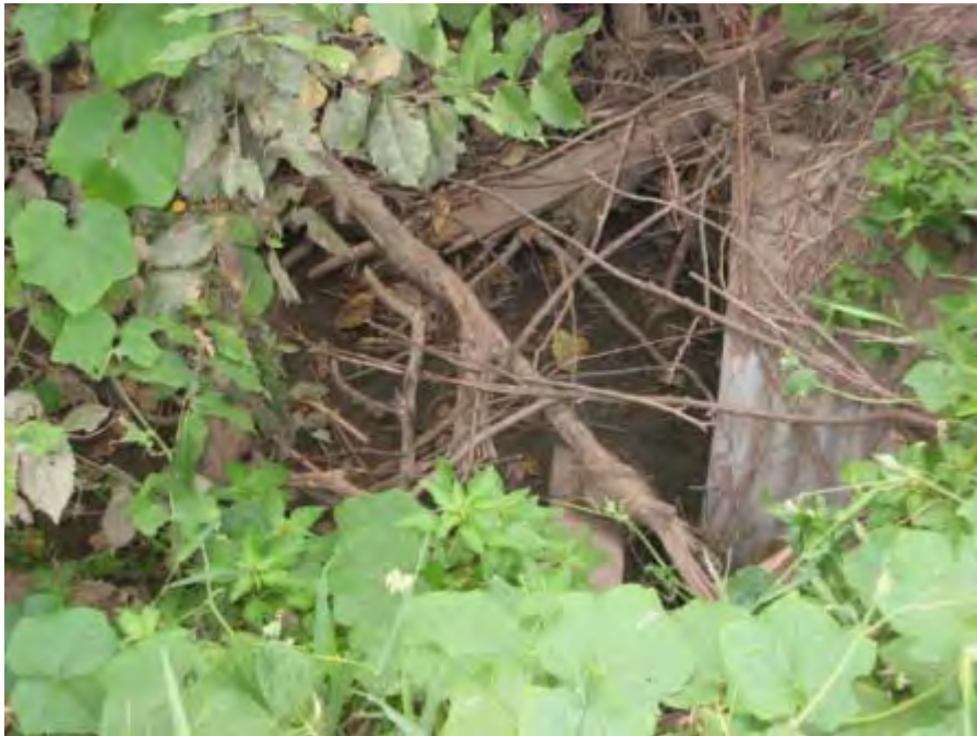
Photo 4. Middle Site - Culvert connecting drainage to Middle Site-3-foot CMP, ½ silted
