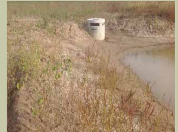
LACK OF VEGETATION
