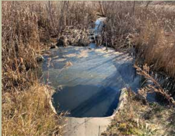
STANDING WATER/SCOUR HOLES
