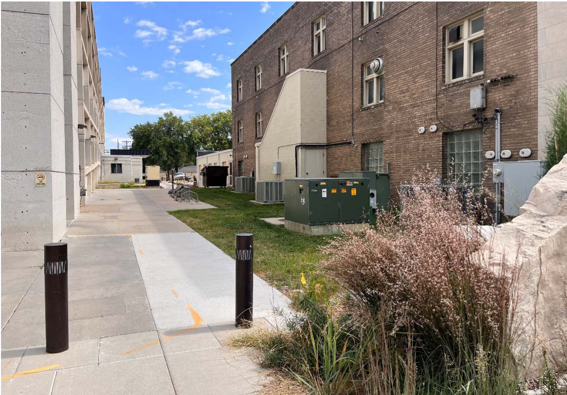
View from Centennial Mall of the existing equipment
