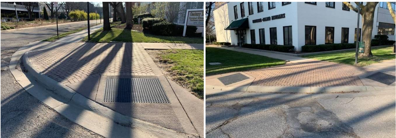
The photographs above show the southwest and southeast corners of Lincoln Mall and S 12 th St. As part of the effort to make the curbs ramps ADA compliant, the paver fields at these corners are proposed to be replaced with grey concrete.
