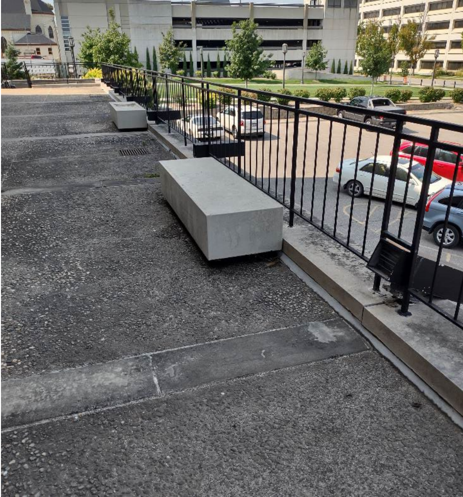
Deteriorating non-ADA-compliant plaza surface, non-compliant railing, joints and sealant
