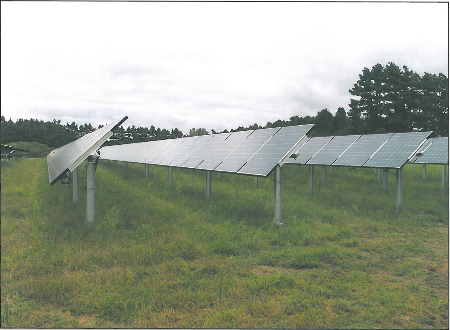
Figure 2: Somers Solar Center (CT) - Solar modules and their racking system. The design of this facility will be very similar to the Holdrege Solar Center in Lincoln, Nebraska.
