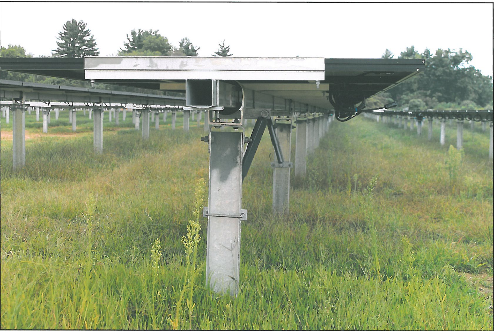
Figure 1: Somers Solar Center (CT) - close up image of single-axis tracking design and racking system. This technology will track the sun on an East-West axis throughout the day.
