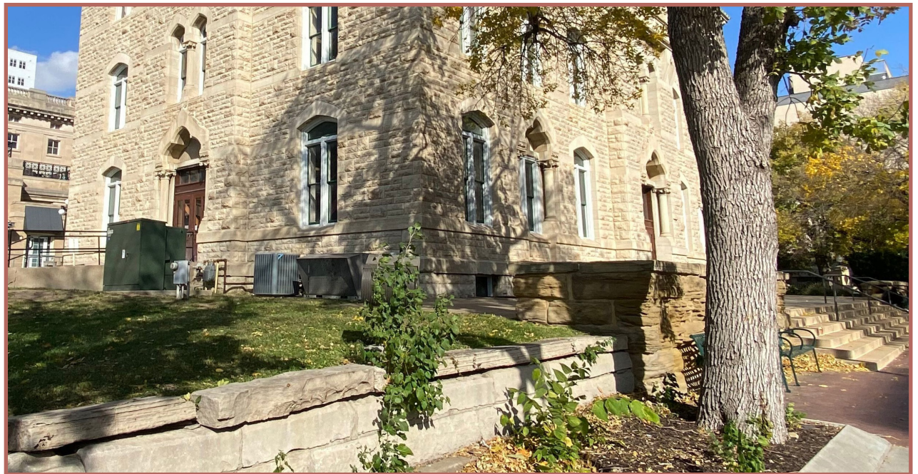
The ground mounted mechanical units at Old City Hall are very large and visible from the public right-of-way and not properly screened with fencing material.
