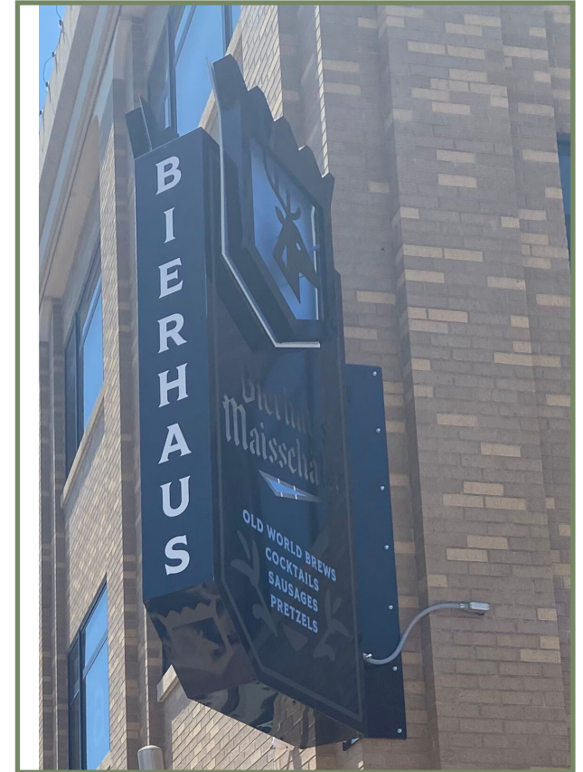
Example of limited amount of conduit and wiring exposed on the building to illuminate the sign.
