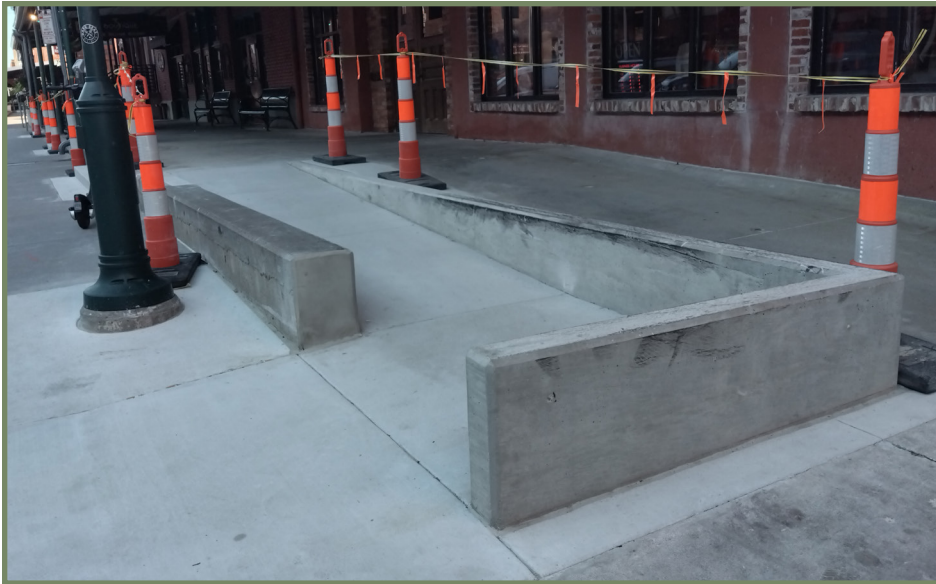
The above ramp was installed to provide ADA access to the businesses in the historic district. The low profile of the ramp walls avoids obscuring the facade of the adjacent historic buildings.
