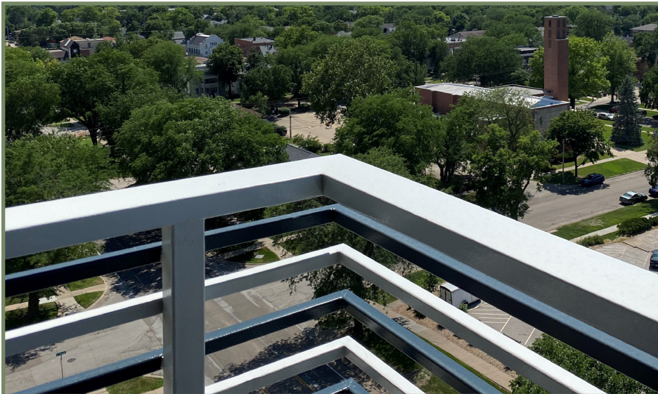
To meet code requirements on guard rail spacing, the Sky Park Manor project added the additional horizontal black rails which fade into the background, allowing the original aluminum rails to stand out.
