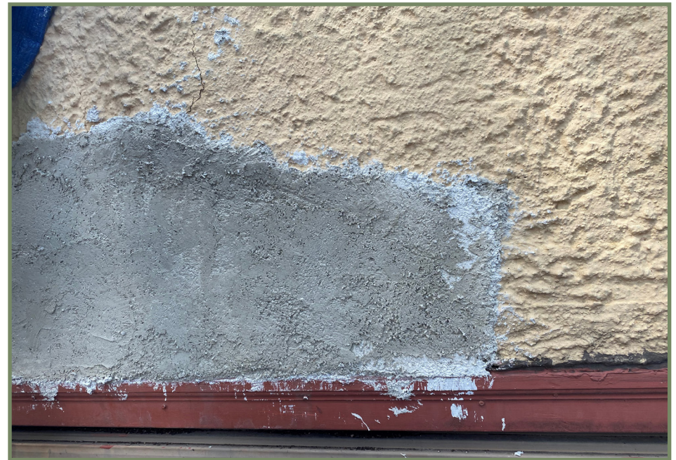
The image above shows a proper patch for an original stucco wall just before painting.
