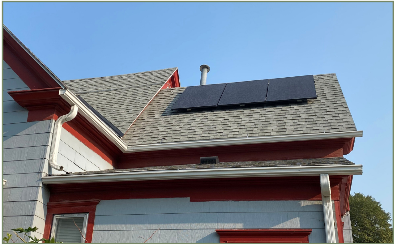
Solar panels mounted with a low-profile, flush against the slope, on a secondary slope.
