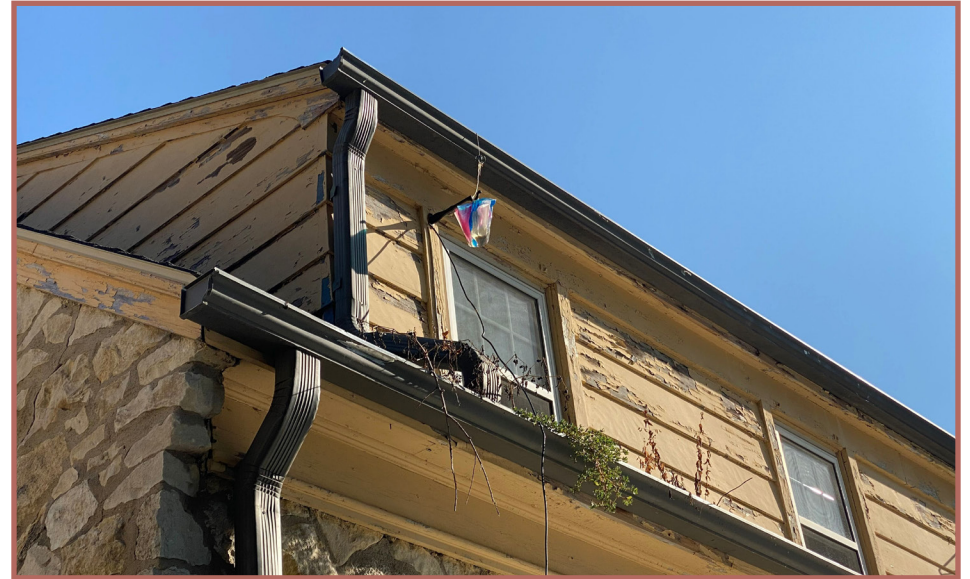
Improper maintenance of gutters which creates risk for water infiltration into the foundation
