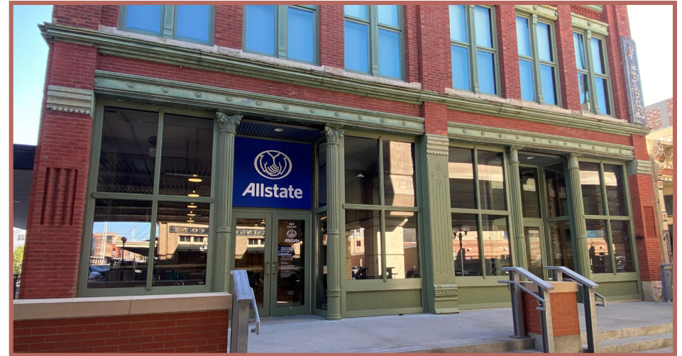
The 1884 Schwarz Paper Building at 747 O Street features a cast iron storefront with engaged Corinthian colonettes, central pier, rosettes and terra-cotta capitals.
