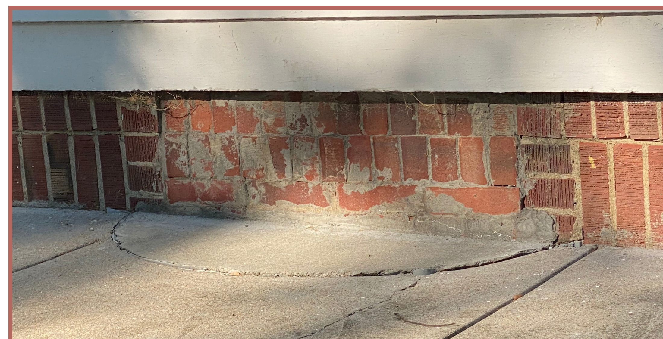
Improper blocking in of basement window
