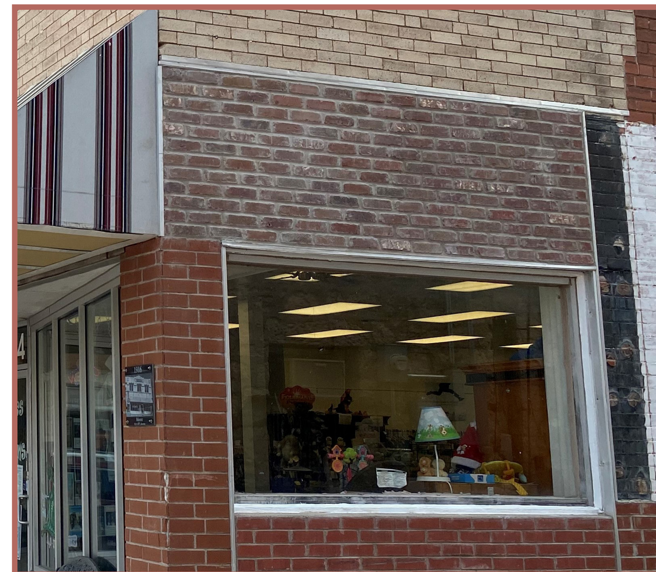
The example above should be avoided as the repair and replacement of brick over time has used three different bricks along with painted brick creating a mismatched appearance.
