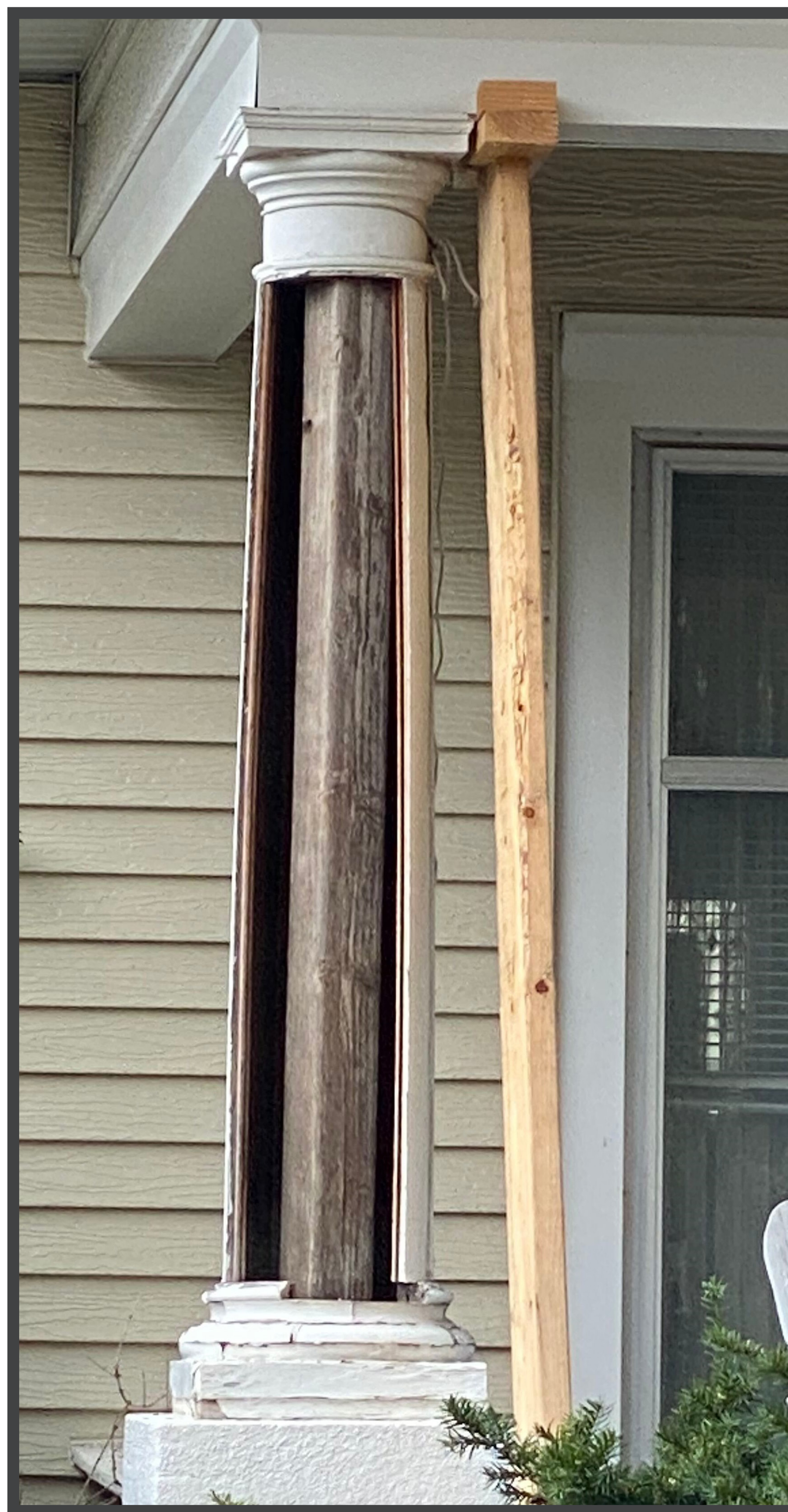
The example to the left shows a rounded column exposed to reveal the true 4x4 structural post supporting the front porch. Alterations that require new structural reinforcement should replicate the original column surround.
