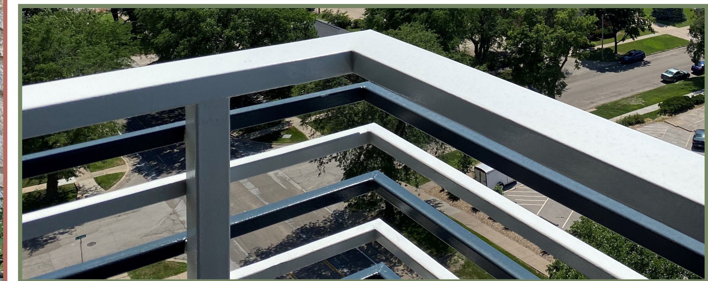
To meet code requirements on guard rail spacing, the Sky Park Manor project added the additional horizontal black rails which fade into the background, allowing the original aluminum rails to stand out.
