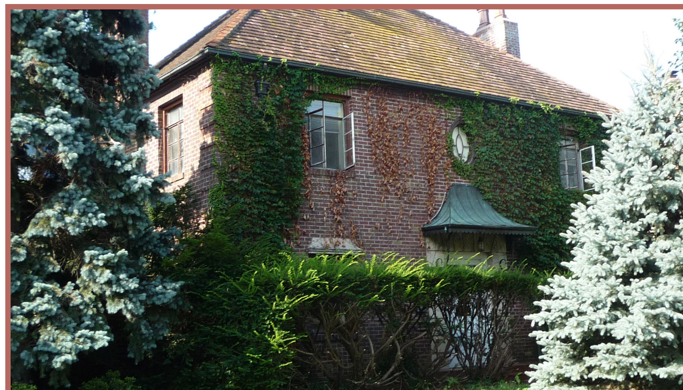
The landscaping has grown to a height that obscures first floor windows and the vines are growing over second floor features.
