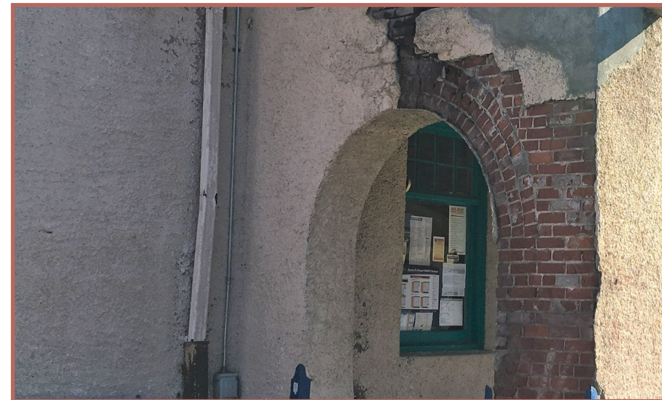
An example of a brick structure once covered in stucco that is failing and breaking away. In this case, the stucco should be carefully removed and the brick and mortar repaired.
