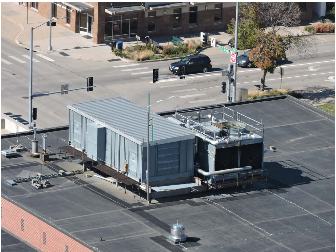
The above image offers a mocked-up look at the approximate location and scale of proposed antenna to be placed on the rooftop of 501 S 14 th Street.
